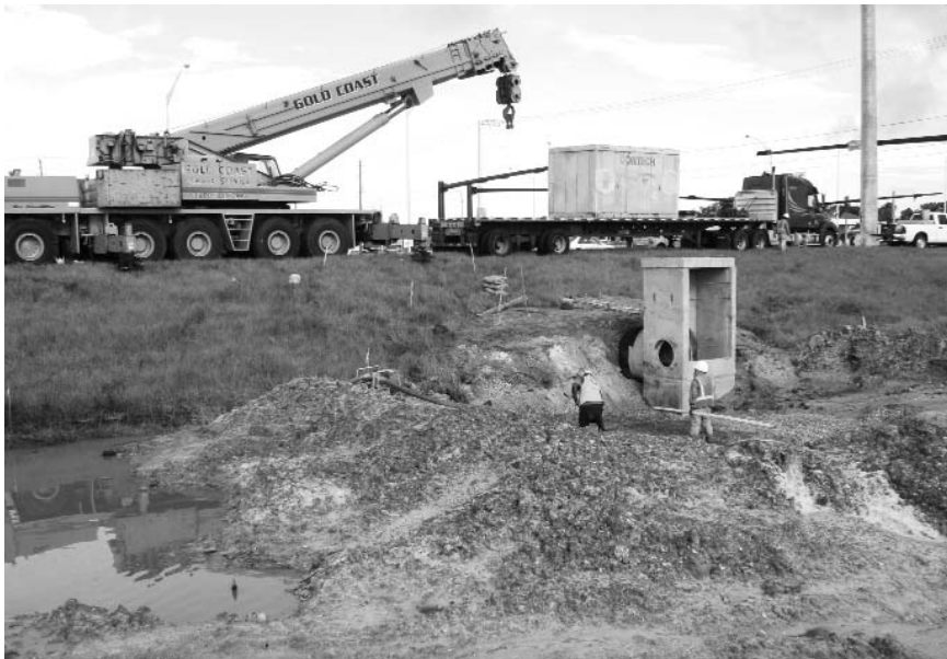
Retrofit of Pond No. 3 with a hydrodynamic separation device (on truck) and control structures to improve water quality from US 441 to the proposed chambers
