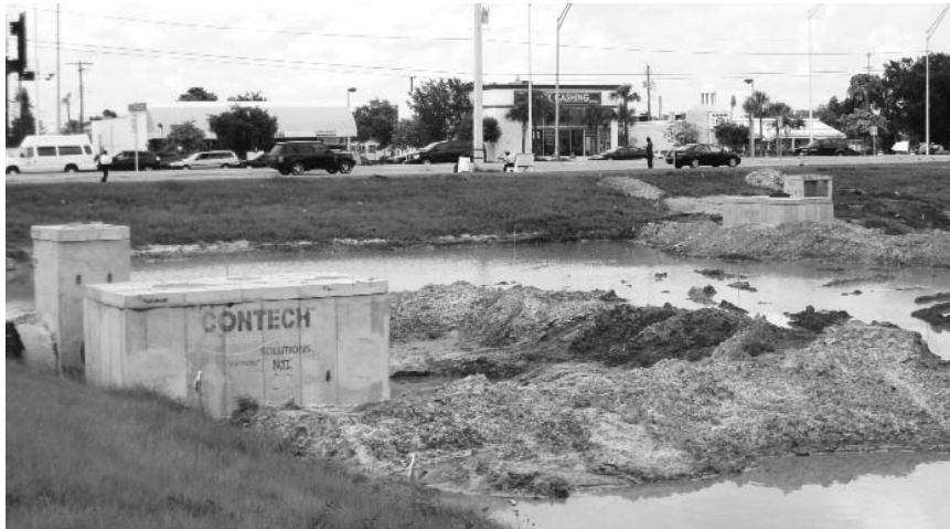
Completed Pond No. 5 Phase I with two hydrodynamic separation devices and two control structures located at Hallandale Beach Boulevard and US 441.
