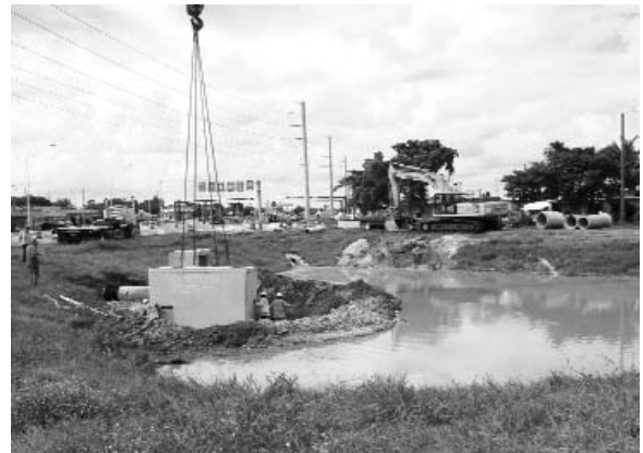
Positioning a hydrodynamic separation device on the east side of US 441, which will be followed by the installation of chambers in Pond No. 4.
