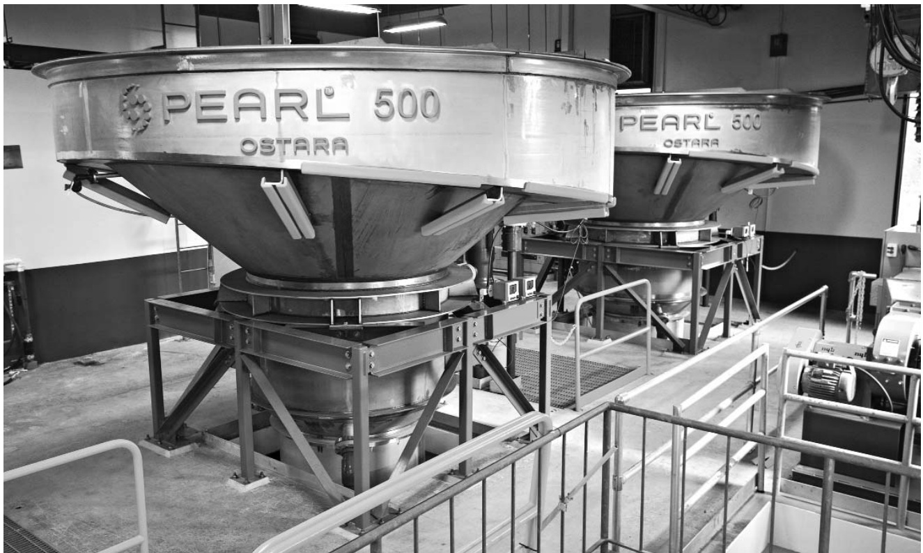
The Durham Advanced Wastewater Treatment Facility is the first commercial facility in the country to incorporate the Pearl® Nutrient Recovery Process from Ostara Nutrient Recovery Technologies.
