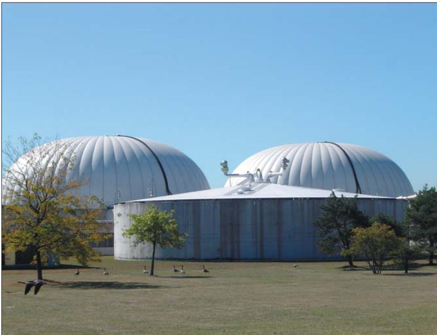
An anaerobic digester with a Dystor® dual-membrane gas holder cover allows gas production to be balanced with consumption.
