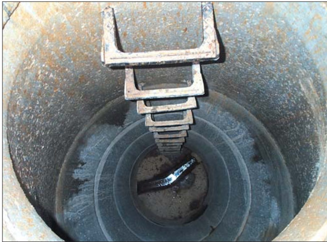
Manhole inspection can reveal defects that may be a major source of infiltration and inflow in a utility's collection system.
