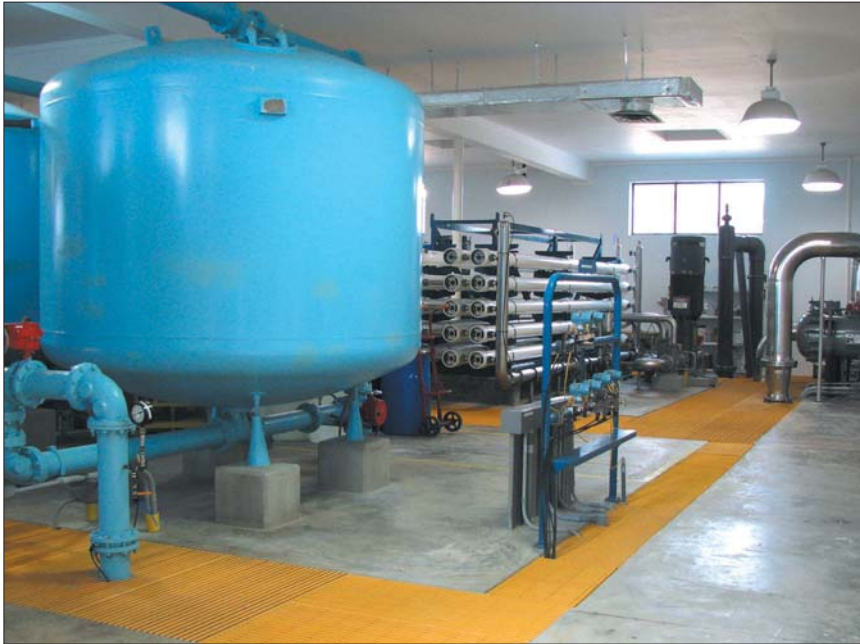
The combination RO/anion exchange plant's output is a blend of RO water that derives from four brackish wells, at an average RO exit flow of 800 gpm, with anion water that derives from 19 freshwater wells, at an average anion exit flow of 200 gpm.
