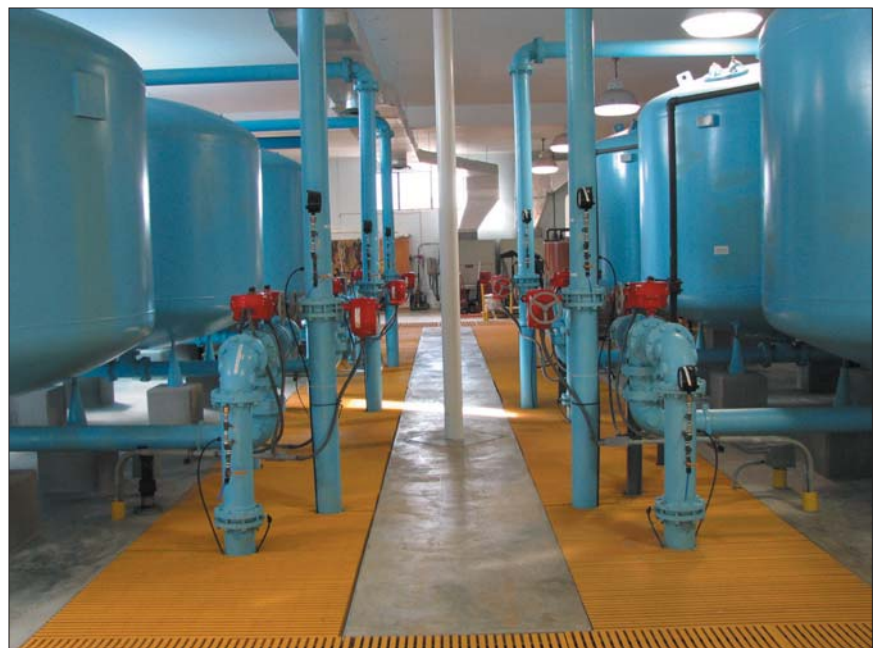
Two 275-cu ft columns of resin handle a service flow rate of two to three gpm/cu ft. Throughput is 14,500 gal/cu ft.
