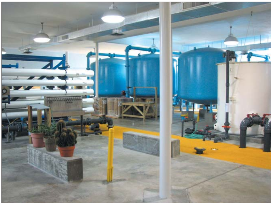
Anion-treated fresh water increases hardness of RO-treated brackish water to both reduce corrosion and help reach the required flow of two mgd. Available fresh water was otherwise not usable for that purpose due to high TOC content.
