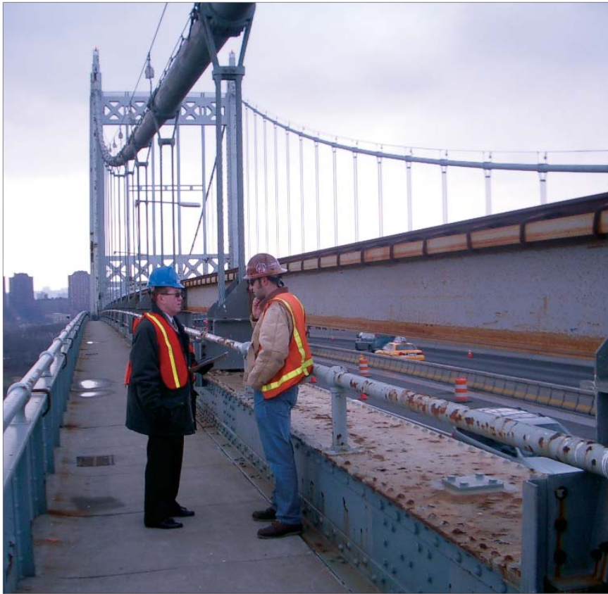
As the Triborough Bridge renovation project draws to a conclusion, galvanized steel median barriers are being placed.
