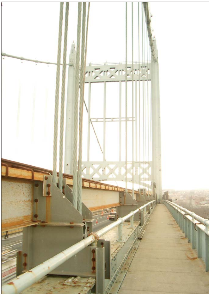
New York City's Triborough Bridge has been undergoing a $550-million renovation program since 1997.
