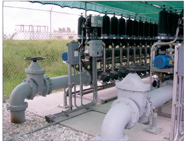
Intake water piping to Turbo-Disc system with booster pumps.
