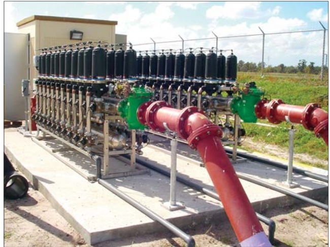
Outlet water piping from Miller-Leaman's 1,400-gpm Turbo-Disc Filtration system.
