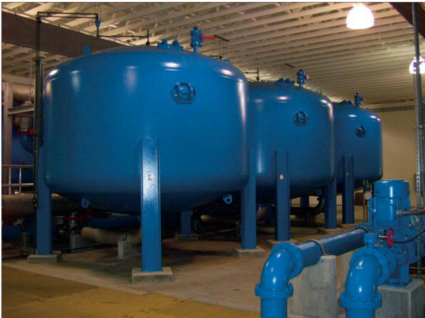
Adsorption system consists of six contactor vessels, configured with three in parallel and then placed in series with a second set of three contactors.
