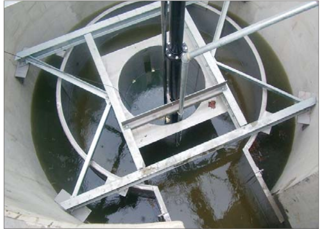
This hydrodynamic vortex separator removes fine sand from the wastewater flow at the Marine Corps Air Station in Cherry Point, NC.
