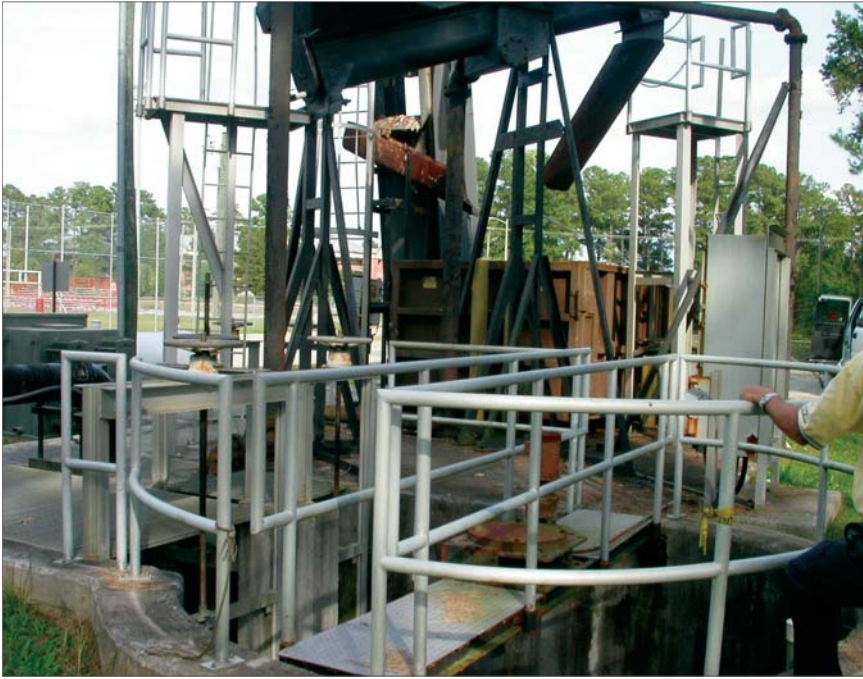
The contractor was able to use the empty chamber of the former grit removal system once all the components had been removed.
