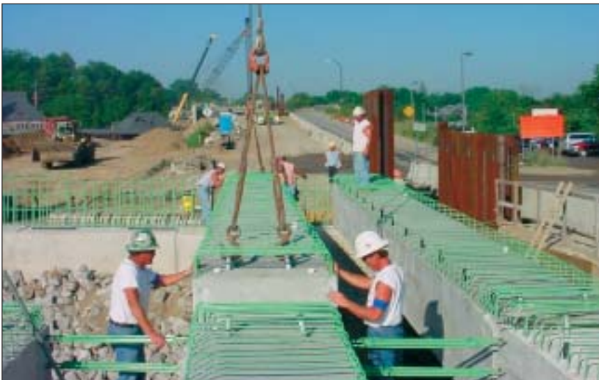
New prestressed, precast concrete box beam bridges replaced two bridges in Ann Arbor.
