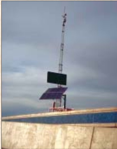
Solar-powered sensors and communication equipment.
