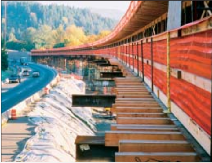
Interstate 90 construction required the use of tight roadway alignments for interchange operations.
