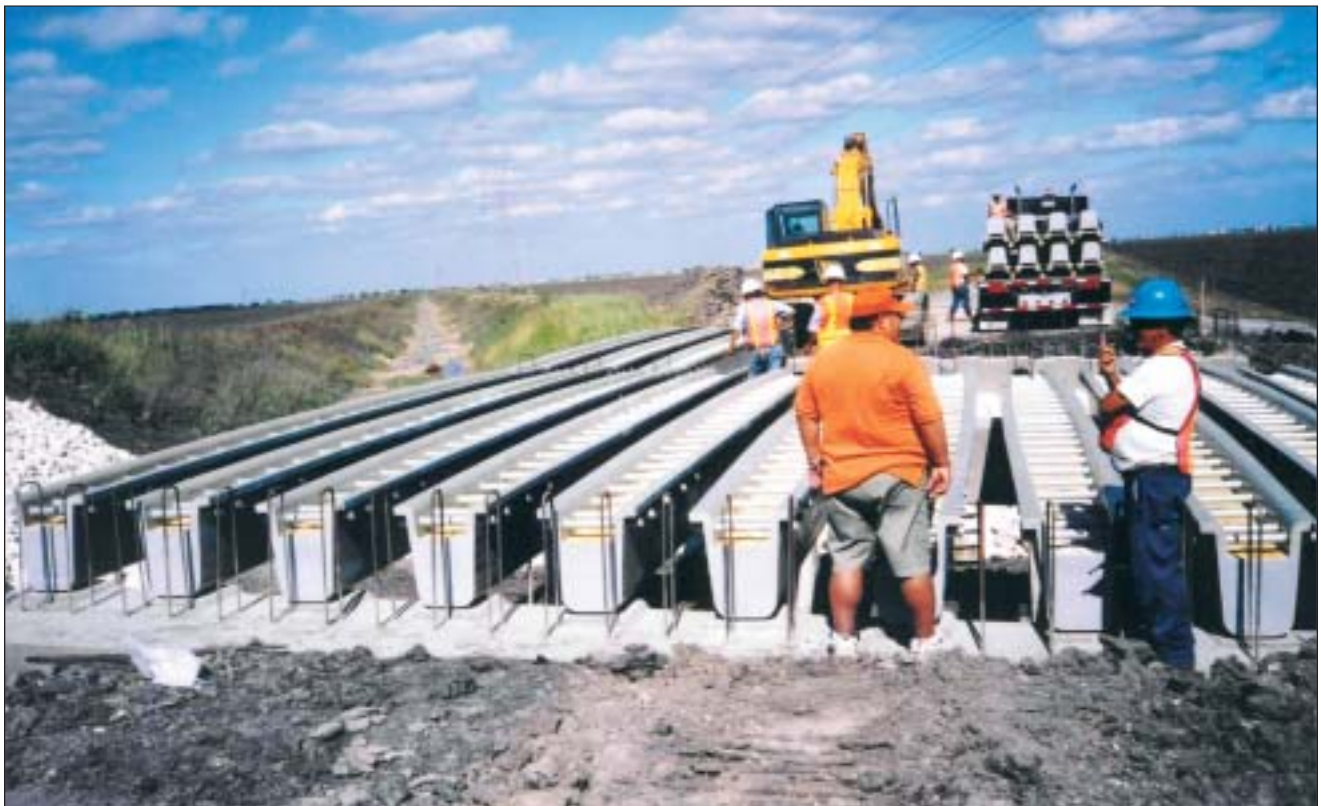
End-on view of U-shaped beams being positioned. The brace bars are visible spanning the open top of the beams.
