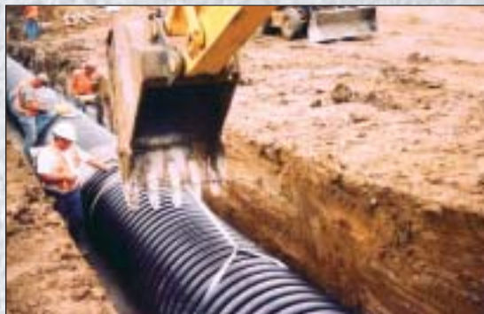
Set for completion in 2006, the expansion of Highway 63 uses corrugated polyethylene pipe for its drainage system.
