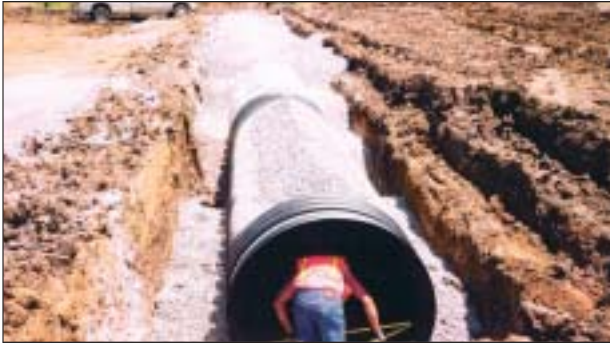
Flowable backfill was used for any pipe installed with less than 32 in. of cover. Backfill consisted of a thin water mix of sand cement poured to one ft above the pipe.
