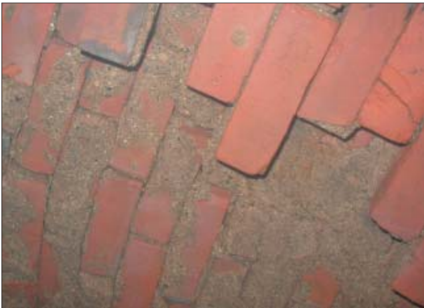
Mortar loss and severe diagonal cracking in the bend were compounded by a 4-ft by 5-ft section of missing blocks.
