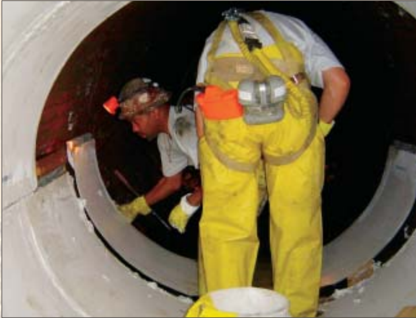
After panels were lowered down the Nelson street shaft they were carried through the sewer and around the 90-degree bend to the designated location under Taylor Street where they were assembled.
