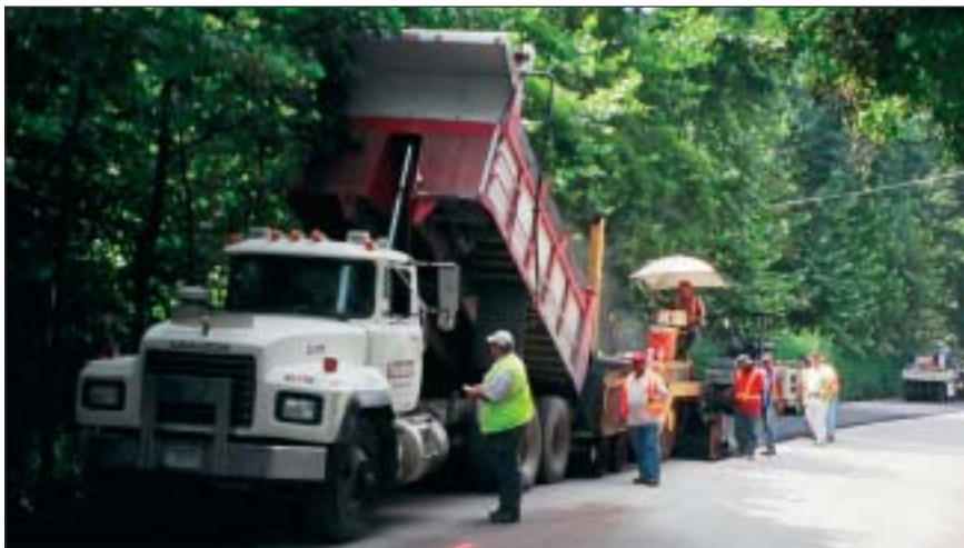
Two in. of black HMA overlay is placed upon a lighter colored five-in. layer of foamed asphalt base. The paint marks denote the centerline of the road. The cold-recycled base resembles that of a high-quality HMA binder mix.
