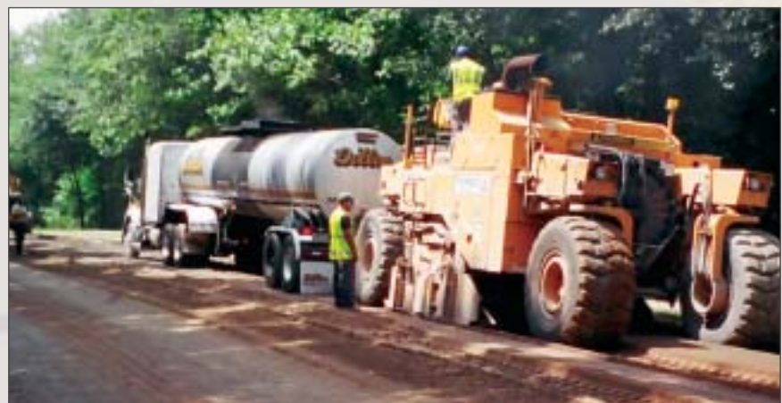
Pulverizers like this one not only grind up the existing roadbase, but they also perform the actual foaming process with specially designed onboard computers and asphalt expansion chambers.
