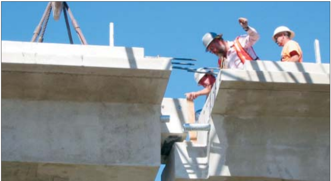
The design team developed a unique precast segmental bridge design that could be erected in one weekend's closure of US 60. After erection, the five superstructure segments were post-tensioned together to form a continuous two-span superstructure.
