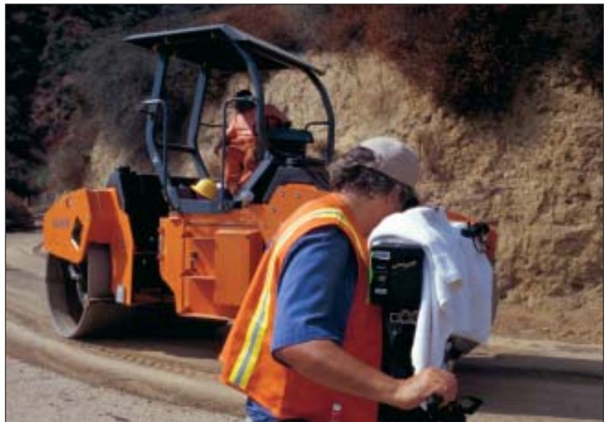
A film crew for The Learning Channel's Monster Machines program videotapes a Hamm HD 120 double-drum vibratory compactor hard at work on Mt. Lee Drive.
