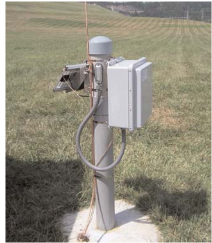
The ADAS consists of 81 vibrating-wire pressure transducers being read by Campbell Scientific CR1000 dataloggers and 25 AVW206 wireless interface units.
