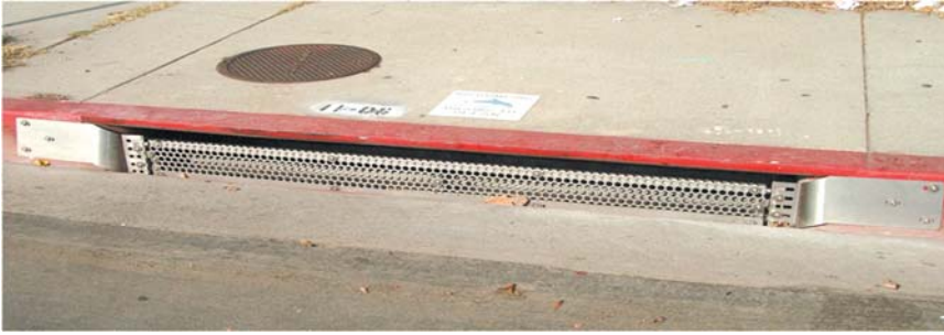
Catch basin inserts and covers, installed in three phases. Phase 1 (completed): 8,000 inserts and 6,000 screens installed to achieve 20 percent trash reduction in the Ballona Creek and Los Angeles River watersheds. Phase 2 (completed): Installed 6,400 screens to increase trash reduction from 20 percent achieved in Phase 1 to 30 percent in the Ballona Creek and Los Angeles River watersheds. Phase 3 (in progress): Installation of 34,000 more catch basin screen covers.
