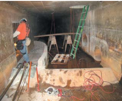
Upgrades are being made to an existing stormwater double-box culvert to allow dry weather flows into a low flow diversion unit in the Pacific Palisades.
