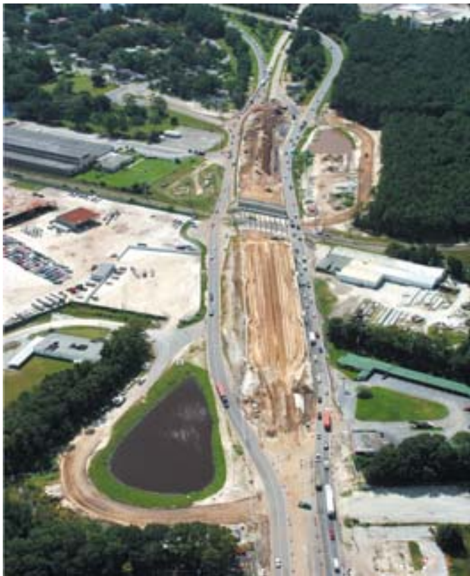
Program management enabled the Better Jacksonville Plan to combine roadway and utility projects to streamline design and construction. Photo courtesy of www.aerophoto.com.
