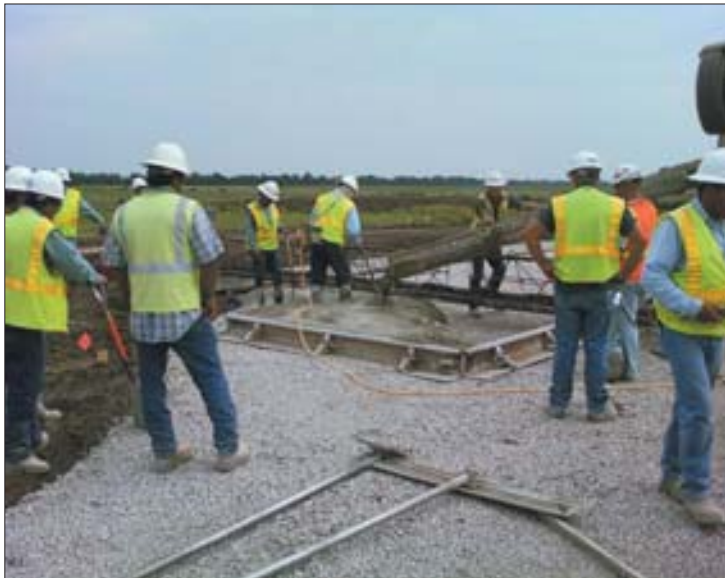
All construction materials were to be non-metallic to maintain a magnetically free site, so fiberglass dowel bars were used to transfer loads between concrete panels.
