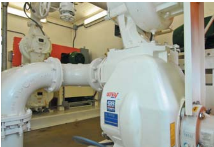
By using the Ultra V, the WCRSA was able to reduce the pump's required footprint while further maximizing the new pump station's overall efficiency and performance.
