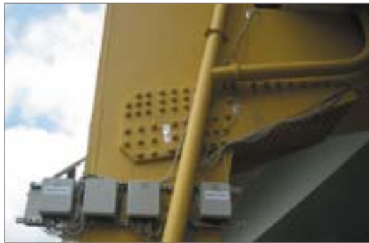
Strain gauges provide real-time information about the loads and stresses on the Tobin Memorial Bridge.
