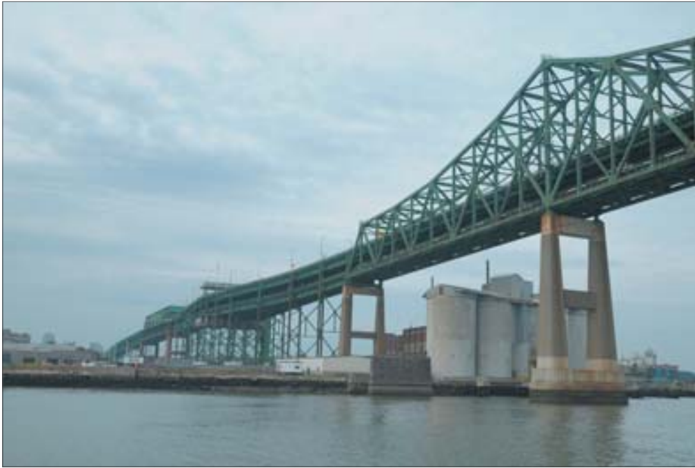
A major link between Boston and northern New England, an estimated 26 million vehicle trips are taken over the Tobin Bridge annually.
