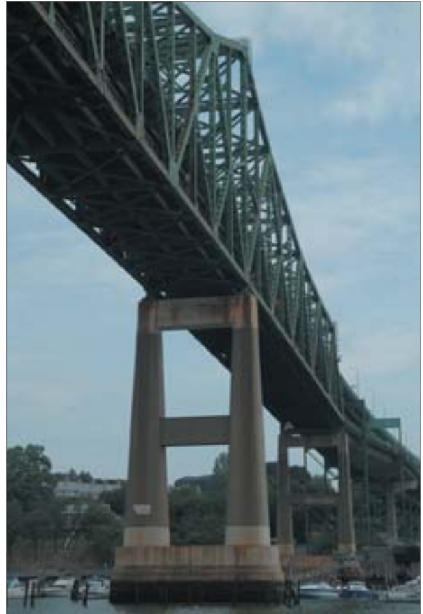
Piers in the Mystic River are anchored as deep as 85 ft below sea level. The tallest measures 339 ft from top to bottom.
