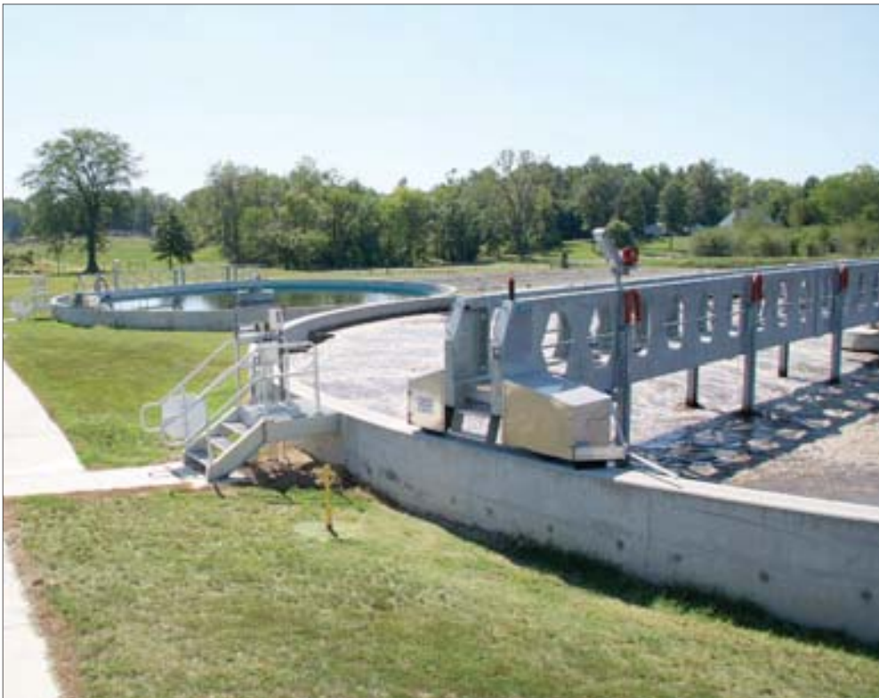
The moving bridge at three ft/second mixes the complete aeration reactor. Only the air needed for the biological process is supplied through fine bubble diffusers.
