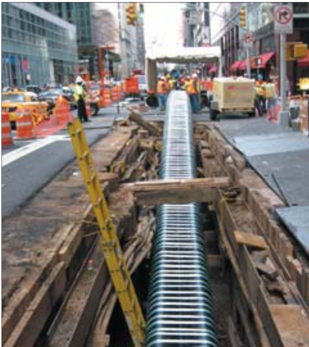
Folded and banded in place with plastic straps, the pipe is inserted into the existing pipe where it will be filled with water and pressurized to snap the straps.
