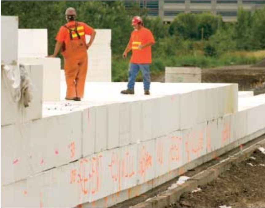
Assembly of the geofoam on the west approach embankment was likened to “putting together a giant, three-dimensional jigsaw puzzle.” Photo by John Livzey.
