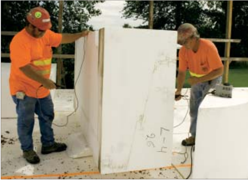
Geofoam was cut by two men using an electrically heated wire about five ft long. Photo by John Livzey.
