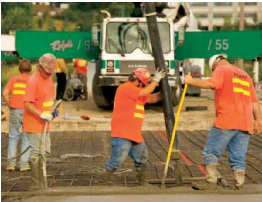
A six-in. thick reinforced concrete slab was poured on top of the geofoam to protect it from solvents and provide lateral support for concrete panels intended to cover the embankment. Photo by John Livzey.
