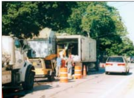
Ingenuity and planning combined in Mansfield, MA, to produce a cost-effective program for eliminating I/I.
