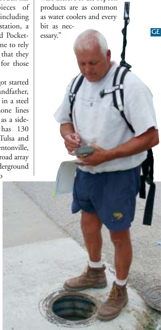
Don Shope uses a Topcon GMS-110 GPS unit and FC-100 data collector to record information on a water meter location for Tulsa. Shope is an employee of Keystone Plumbing, a subcontractor to W. N. Couch.
