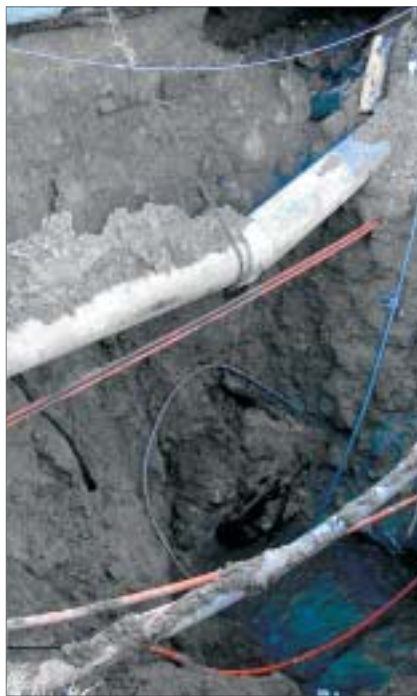
The Essen Lane collapse exposed the failure in the top of the 54-in. RCP sanitary sewer gravity main. At the top, a 15-in. potable water main is broken and numerous other utilities are adjacent, including telephone, cable, and fiber optic lines.
