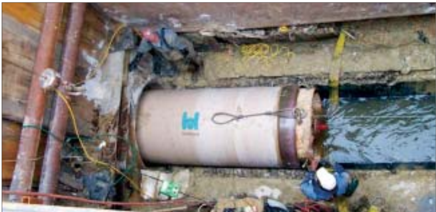
Allen & LeBlanc crew members slipline the 48-in. CCFRPM pipe into position. The integral fiberglass low profile bell is gasketed and provides a watertight seal with the spigot joint while allowing the pipe to be pulled or jacked into the host pipe. The low profile design prevents hang-ups and minimizes friction during installation. The entire project was approximately 400 ft long.
