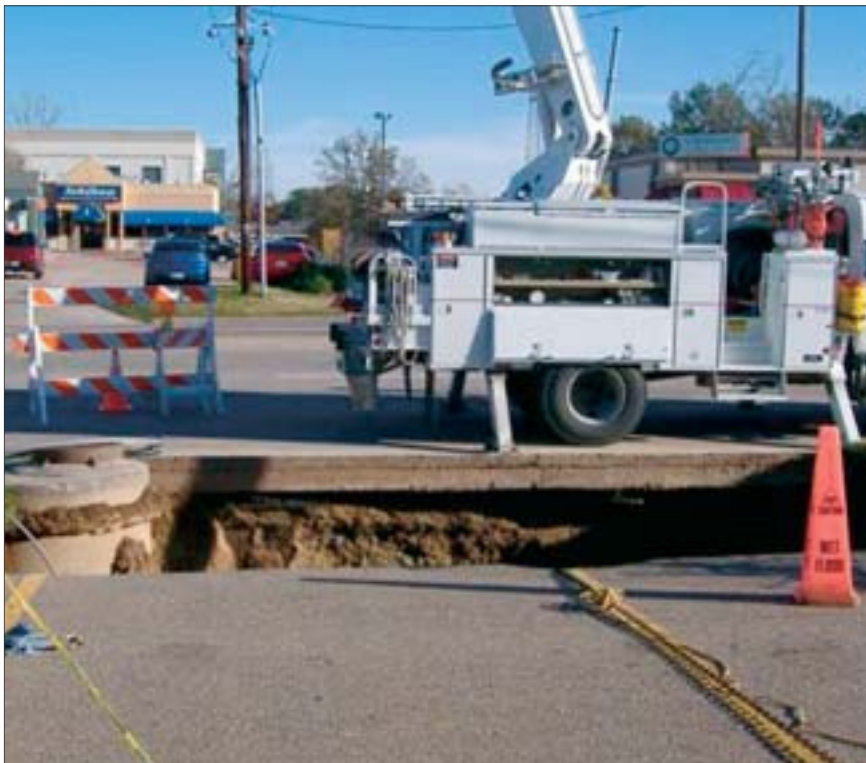
A sinkhole formed in Baton Rouge along the shoulder of Essen Lane, washing out of the area beneath the Albertson's parking lot. A nearby Entergy power pole and several buried utility lines were in danger.
