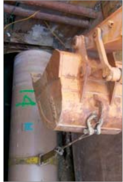
A sling attached to an excavator easily handled a lightweight 20-ft joint of 48-in. CCFRPM sliplining pipe, lowering it into the installation pit.
