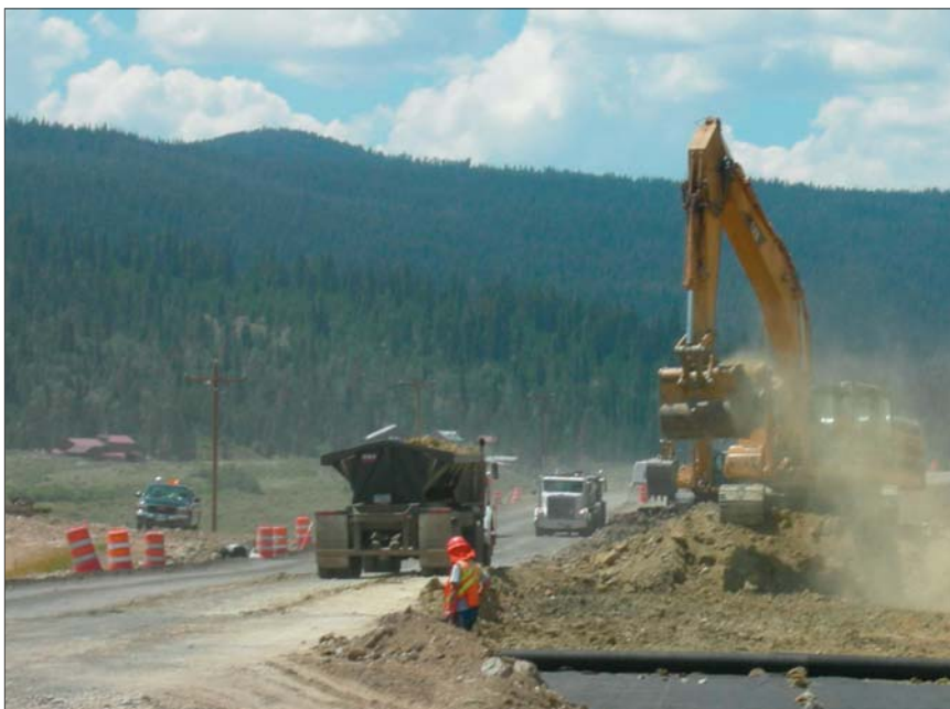
Crews moving dirt and laying out material separation fabric through soft subgrade as part of the preparation to widen the highway on the east end of the Brooks Lake section of The Togwotee Trail corridor. Credit: Wyoming Department of Transportation.
