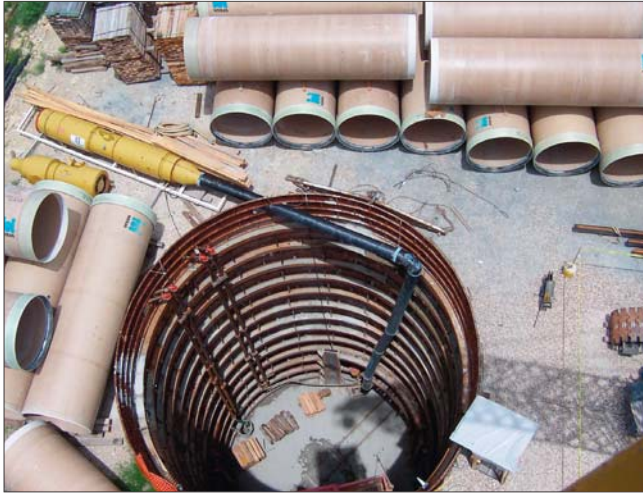
On the Little Walnut Creek project, the design called for inserting 10,000 ft of 60-in. diameter pipe into the tunnel from installation shafts at each end with no intermediate shaft.
