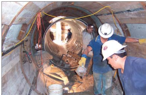
The liner pipe installation was rapid, even through radius curves, due to the lightweight pipe and the push together FWC couplings.
