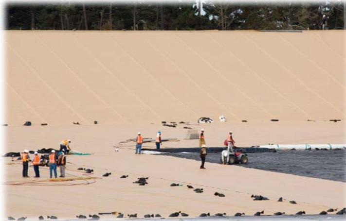
Installation of a high-performance five-ply liner material nears completion at Forest Lake Reservoir in Pebble Beach, Monterey Peninsula, California.
