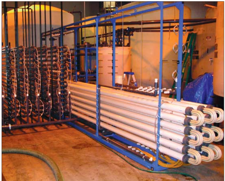
Retrofitting the membrane filtration system with new membranes provided a wider flow channel and better resistance to fouling.
