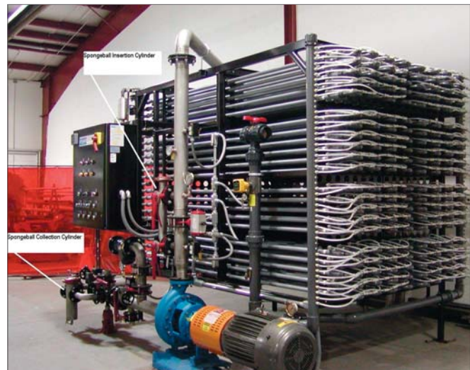
Spongeball cleaning of the filtration system is a mechanical process that reduces both downtime and the consumption of chemicals.
