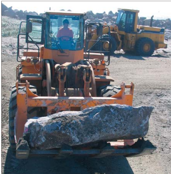
To build a jetty of this type, smaller stones are first placed into a bed of sand, followed by larger core stones.
