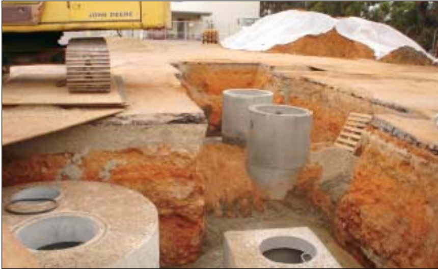
The structure in the left foreground is the opening to the CDS unit. In the bottom right corner of the photograph is the junction/flow control structure. The other two openings provide access to the media filtration device.
