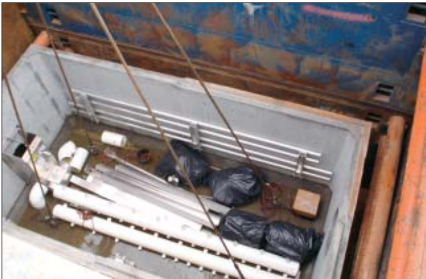
The second half of the treatment train is lowered into place. This 8-ft by 16-ft precast concrete vault contains some of the components that will become the media filtration device.
