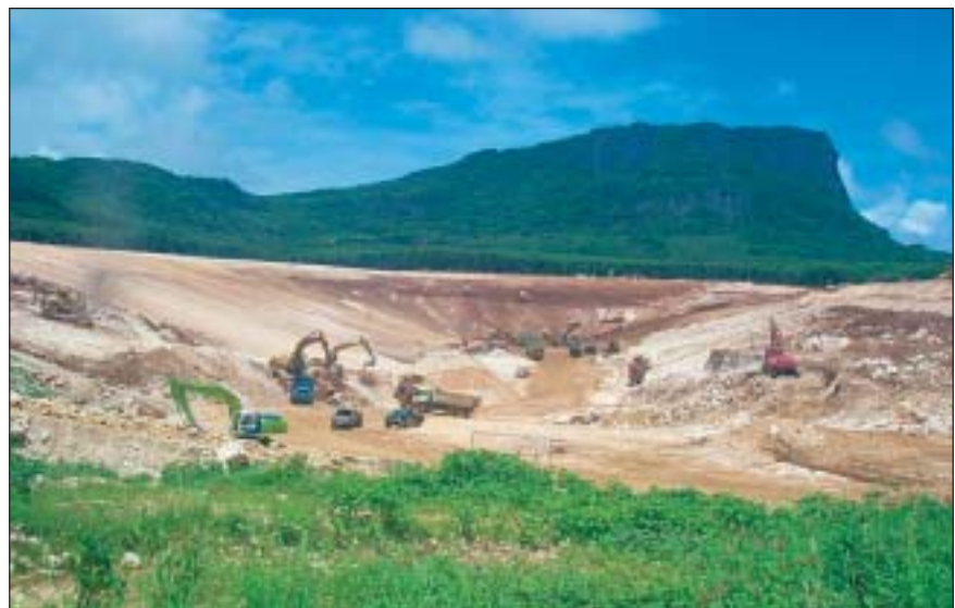
Initial excavation of the lined waste management unit at the Marpi Solid Waste Facility.
