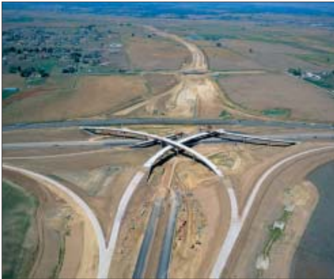
Carter & Burgess provided project oversight engineering services on behalf of the Northwest Parkway Public Highway Authority for the design-build contract of a 9.5 mile toll road north of the Denver metropolitan area. Construction oversight responsibilities included monitoring the design-build contractor's construction progress, their quality control program—including compliance with released-for-construction drawings and specifications—and their quality control and inspection testing activities.
