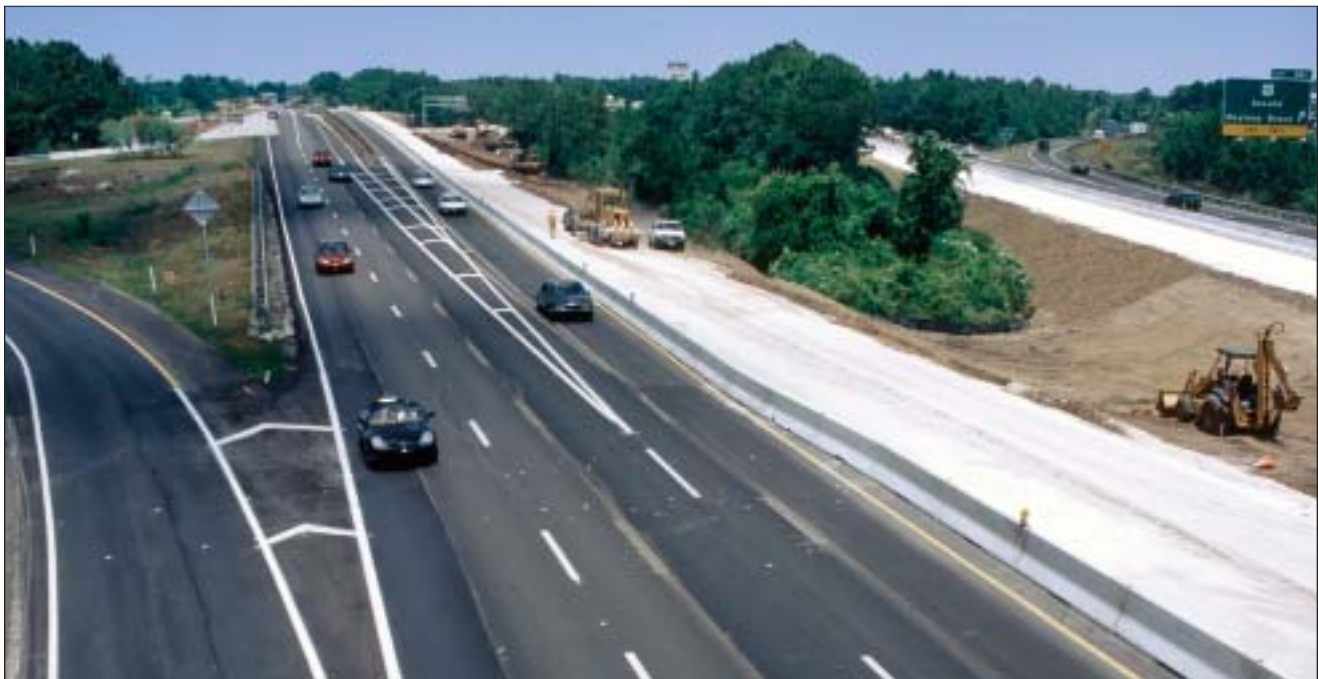
Some projects are ready-made for design build, such as a two-mile widening of Interstate 95 from four lanes to six lanes (three northbound and three southbound). This project also involved the widening of three bridges, drainage, new lighting—including hi mast—upgrades to the ITS system, and reconstruction of 1,000 ft of U.S. 92 under I-95.
