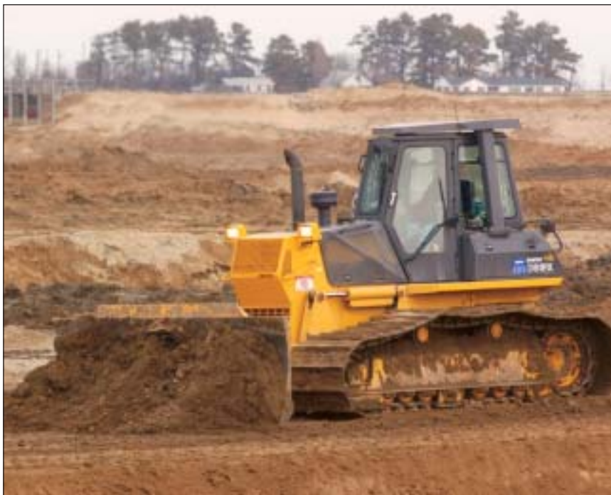
Dozers on Poplar Island are in constant motion shaping and finish grading multiple haul roads located within the borrow pit, a requirement in order to keep trucks on the move.
