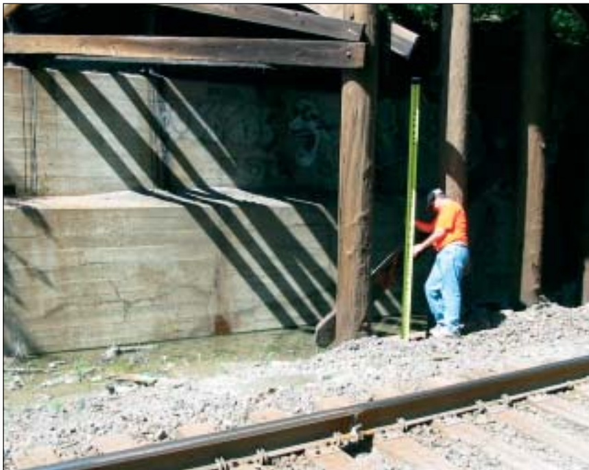
Vertical control being transferred from a monument under a bridge to nearby new "GPS'able" monument by running Second-Order geodetic levels.
