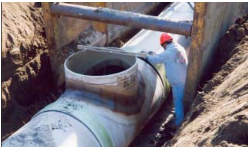
The walls of one of the city's largest sewer outfall lines had corroded from six in. thick to only a few inches. Placement of the new pipe brought city engineers much needed relief from fear of a catastrophic failure.
