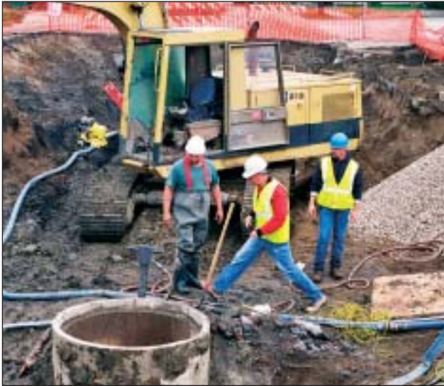
Some innovative project design included leaving joints unsealed on sections of the new storm sewer that went through areas of high groundwater. The effect is to lower the water table and alleviate water problems for property owners.
