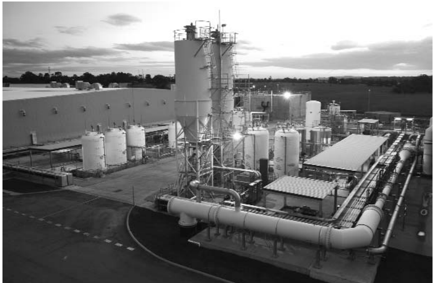
The Bundamba Advanced Water Treatment Plant in Australia is one of three advanced water treatment plants designed to produce purified recycled water from secondary treated water to supplement the region's drinking water supplies if required. (Photo credit: WaterSecure)
