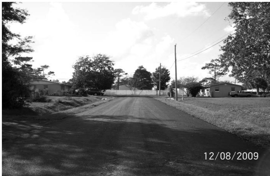
Saracity Gardens today. Drainage was improved by removing trees as required and installing pipes and structures. Sod and asphalt aprons were added once resurfacing of the roads was completed. The Orange County Roads & Drainage Division staff made the needed improvements a reality.
