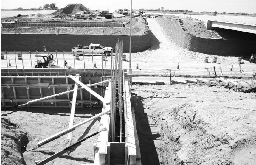
Unique bridge abutment design provides 14-ft maintenance ramp access to I-25 median.
