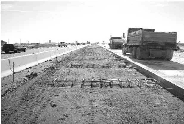
New mainline pavement construction occurred directly adjacent to traffic. Four lanes of through traffic at 65 mph were kept open during reconstruction of the Interstate.
