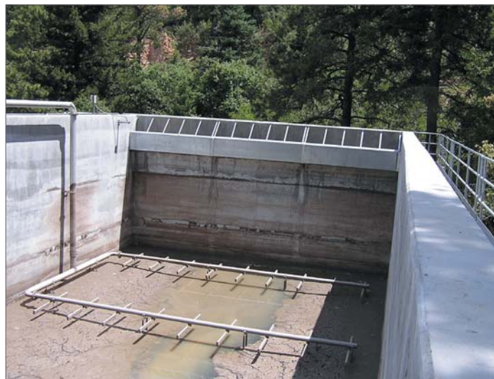
The pre-existing 200,000-gal equalization basin is being retrofitted for the MBR process.
