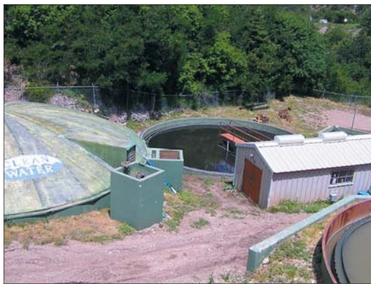
The system employs a second-generation MBR and a gravity-fed RO system to treat wastewater flows that ultimately exceed drinking water quality standards.
