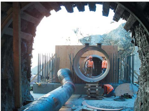
A 505-ft long tunnel in bedrock, which contains 72-in and 24-in conduits, connects the intake to the control house.
