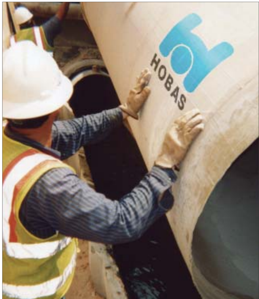
The flush exterior joint and the high-strength yet thin-walled pipe allowed for the greatest flow recovery in the SAWS project. The flow was uninterrupted during the entire sliplining process.
