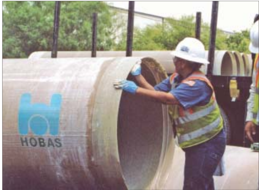
A SAWS worker applies joint lube, the only thing needed to make a quick push-together connection of the pipe.
