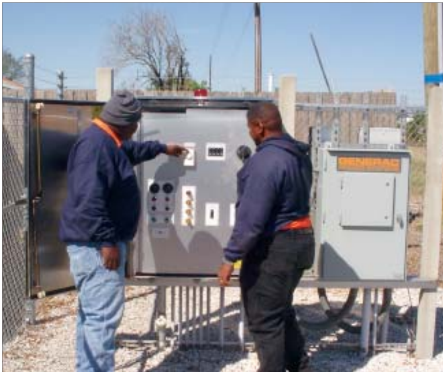
Improved pump controls and the addition of telemetry have improved the operation of Orange County's fixed pump stations.
