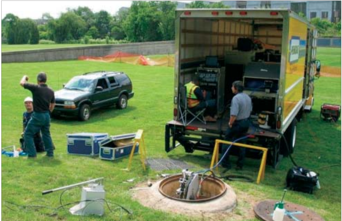
Sahara System set up on the East Side Transmission main in Allentown, PA.
